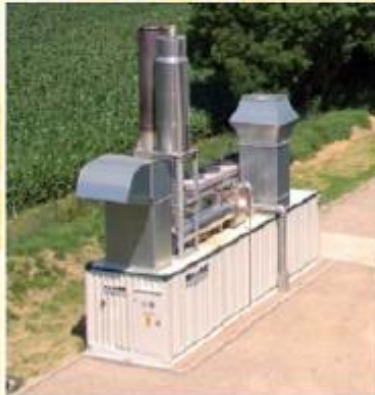
above: The HAASE „Energy Center” container unit also encloses gas cooler, analysis, booster, flare, and the CHP control system.
